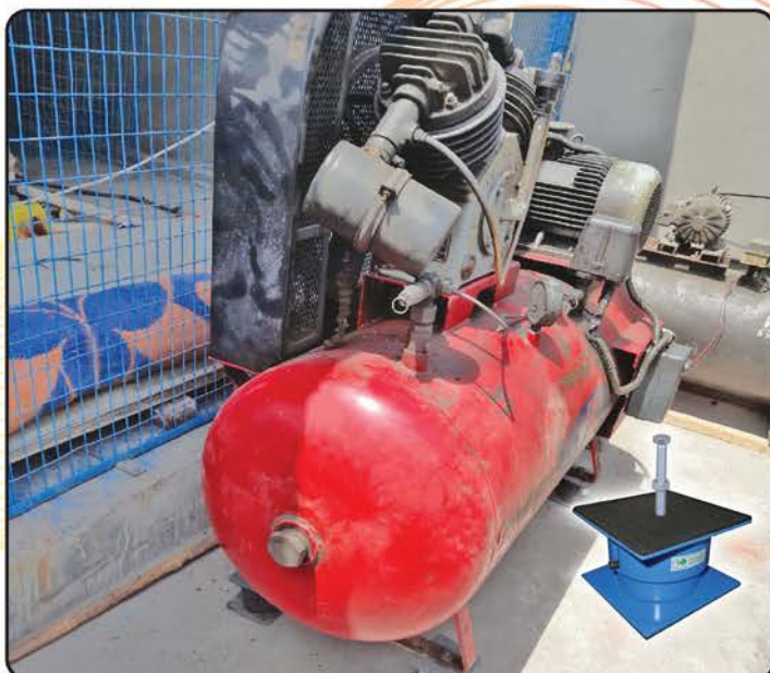
Air Compressor on Single Spring Isolator
