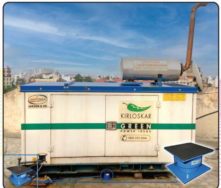
Genset on Dynemech Single Spring Isolator
