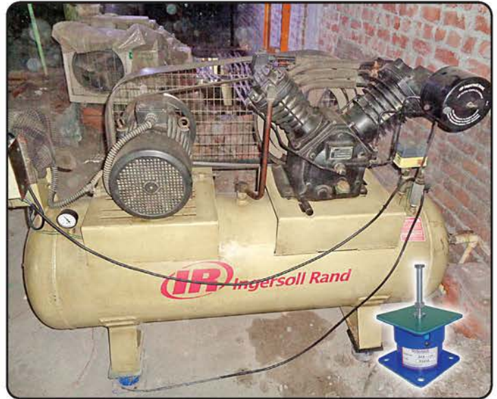
Air Compressor on Single Spring Isolator
