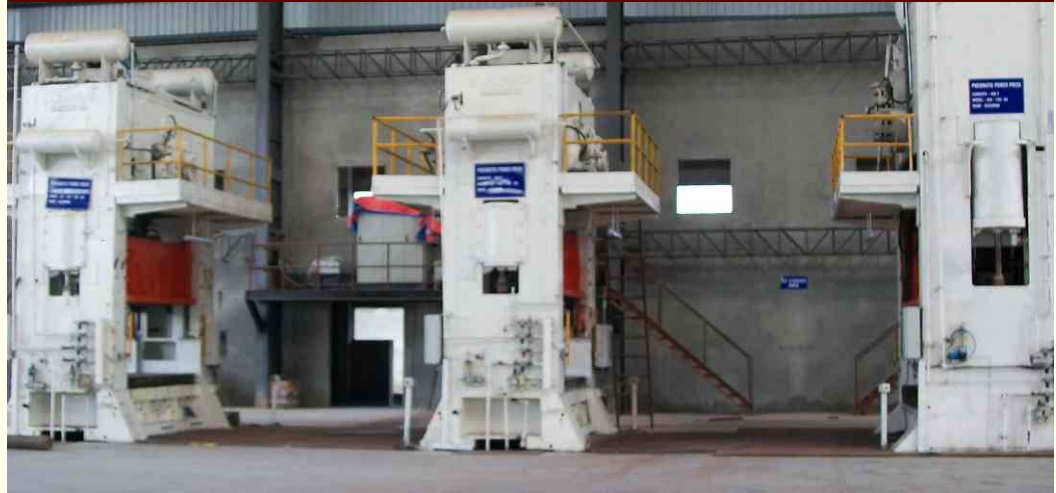
PRESS LINE INSTALLED ON ANTI VIBRATION MACHINE MOUNTS- SPRING ISOLATORS
