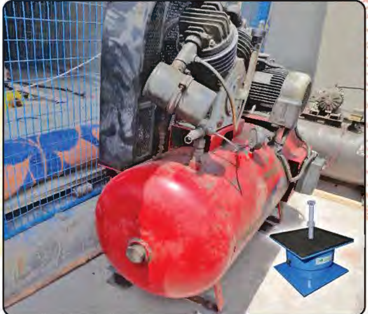
Air Compressor on Single Spring Isolator
