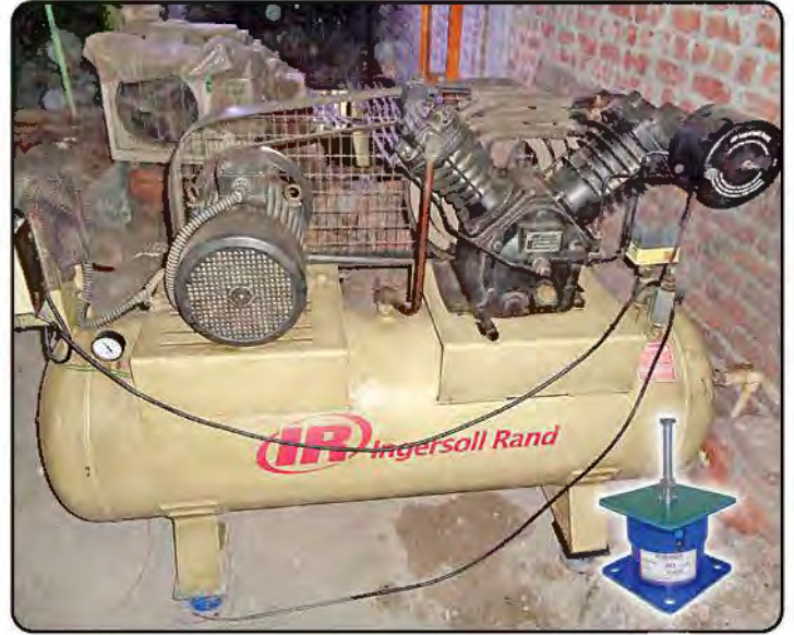
Air Compressor on Single Spring Isolator
