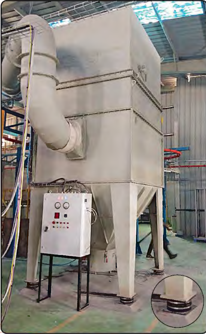
Blower on Suspended Floor on Dynemech Round Spring isolator
